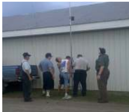
The setup crew works hard to install the HF antenna system for the club booth.
