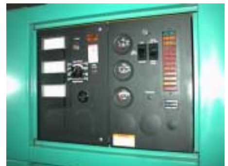
Control panel for the generator at FEMA headquarters
